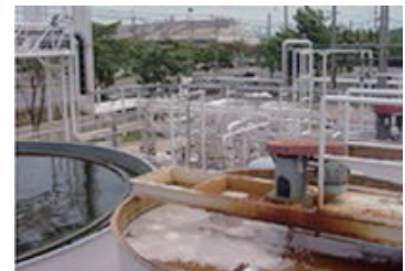
General effluent treatment facilities
