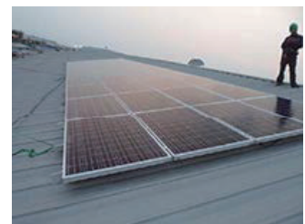
Photovoltaic power generation panels
