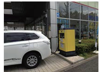
Quick charger installed in a dealer
