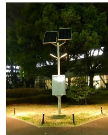
Autonomous street lighting at night
