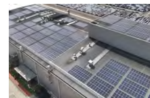
Solar panels on the roof of MMKI's plant
