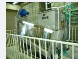
Newly installed screw-type sludge dewatering equipment
