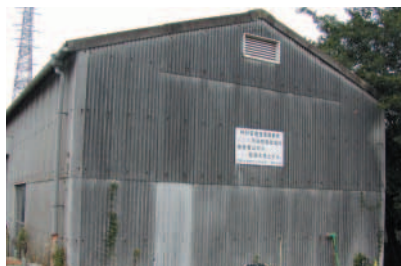
Storage warehouse for equipment containing PCBs
