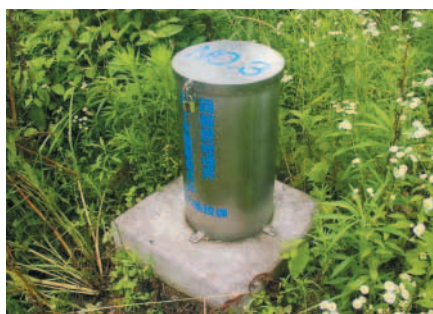
Observation well to monitor groundwater quality
