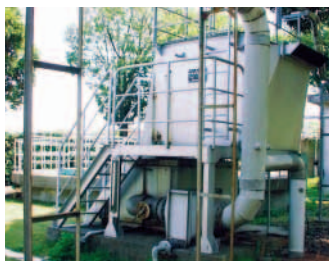
Deodorization equipment at wastewater treatment facility
