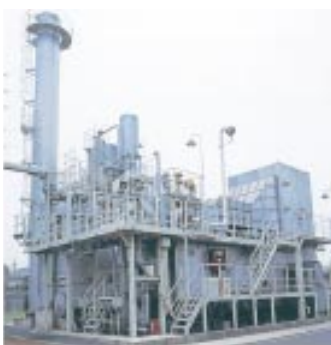
Cogeneration facility at Oye Plant
