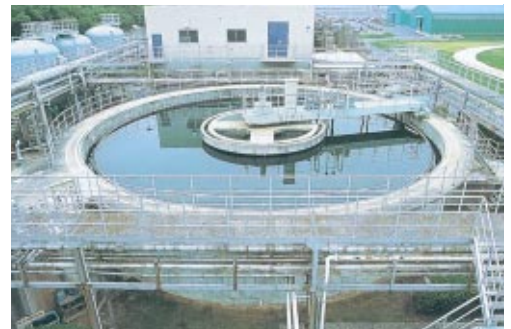
General wastewater treatment facility
